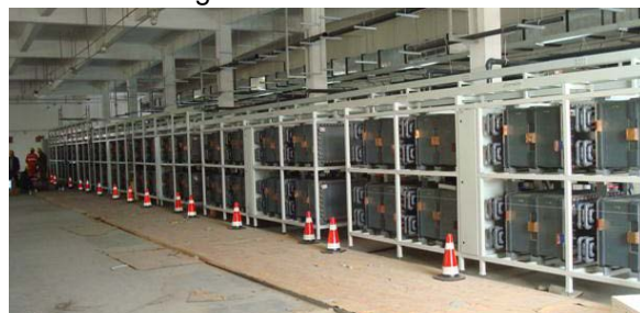
5 MW/10 MWh VRB - Rongke Power - China
